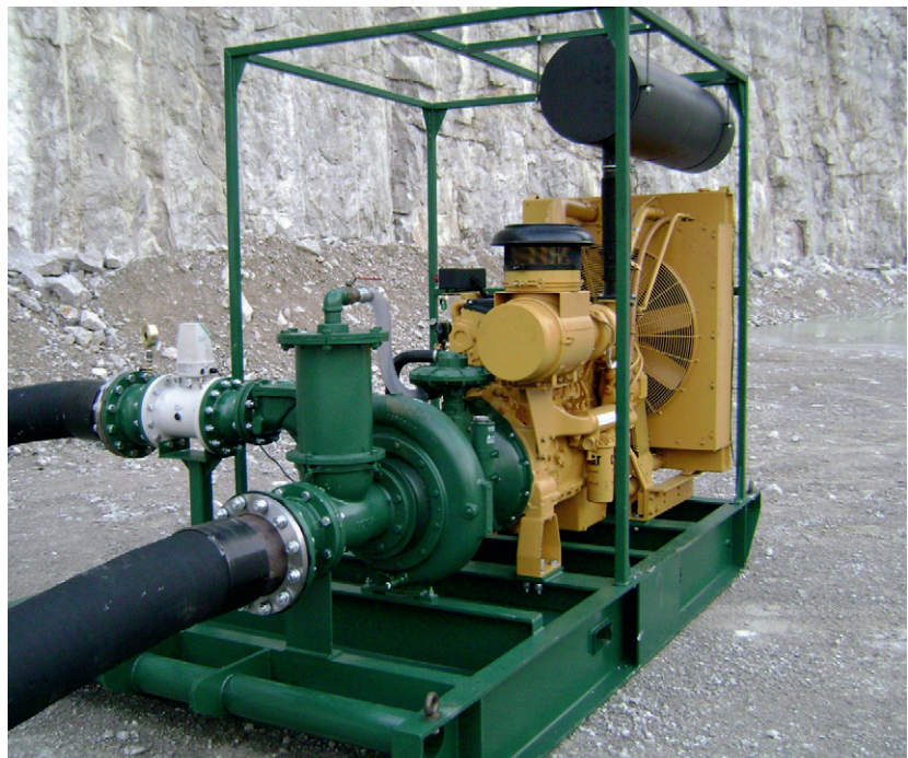
Figure 4. At Halkyn quarry in Wales, a PP108C18 pump is driven by a Caterpillar C15 engine. Sold two years ago, this is still operating today with no need to change the pump. Starting pumping at level 4 of the quarry, it is now on level 7, but will soon have to be upgraded to a pump having a 21 in impeller to accommodate new a duty point.
