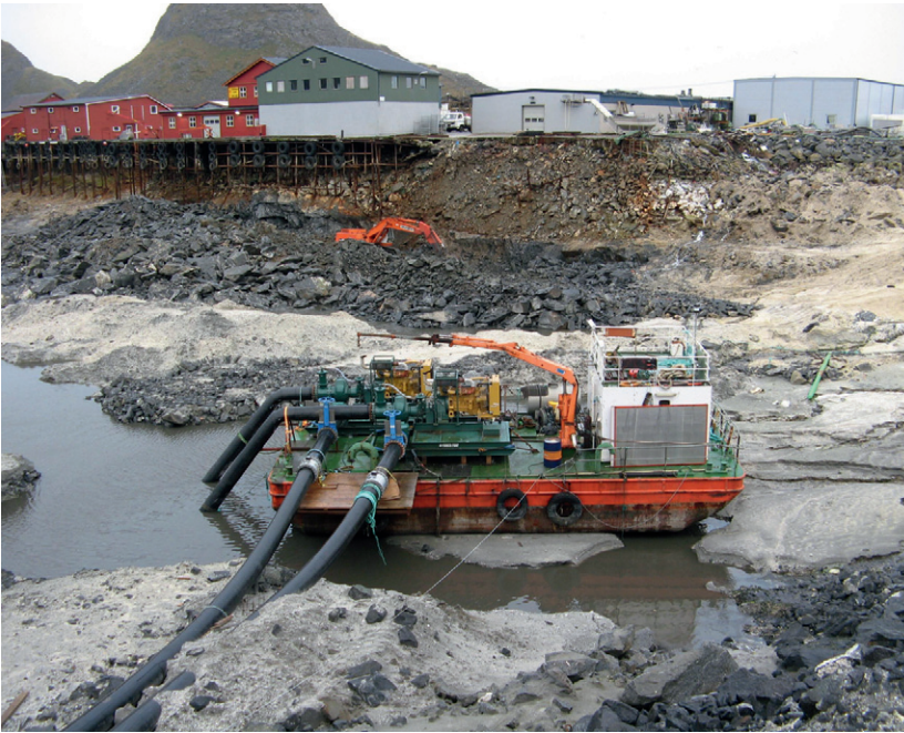
Figure 2. Mounted on a barge, two 18 in pumpsets fitted with 450SM pumps and powered by Caterpillar C15 engines are seen de-watering a Norwegian harbour at a pumping rate of 3000 m 3 /hr at 18 m total dynamic head (TDH).
