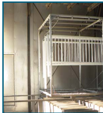
The owners of AR Iron invested in an energy-efficient batch oven with an enlarged opening to accommodate oversized parts.
