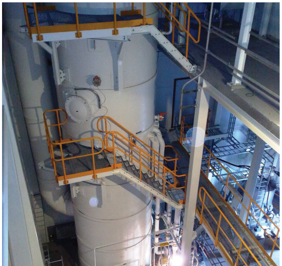
Figure 3: Sulphur dioxide cleaning system supplied to Volvo Powertrain Corporation's foundry in Skövde, Sweden. (Courtesy of Götaverken Miljö AB.)
