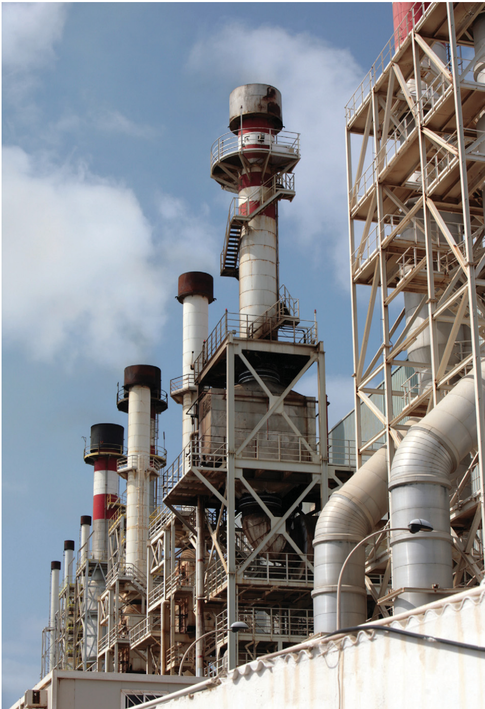
There are many issues involved in selecting pre-treatment technology for desalination in seawater reverse osmosis applications.
