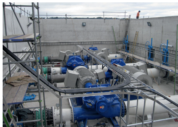
Installing the pumps in the purpose-built structure which has been designed to prevent the incursion of water even in flood conditions.
