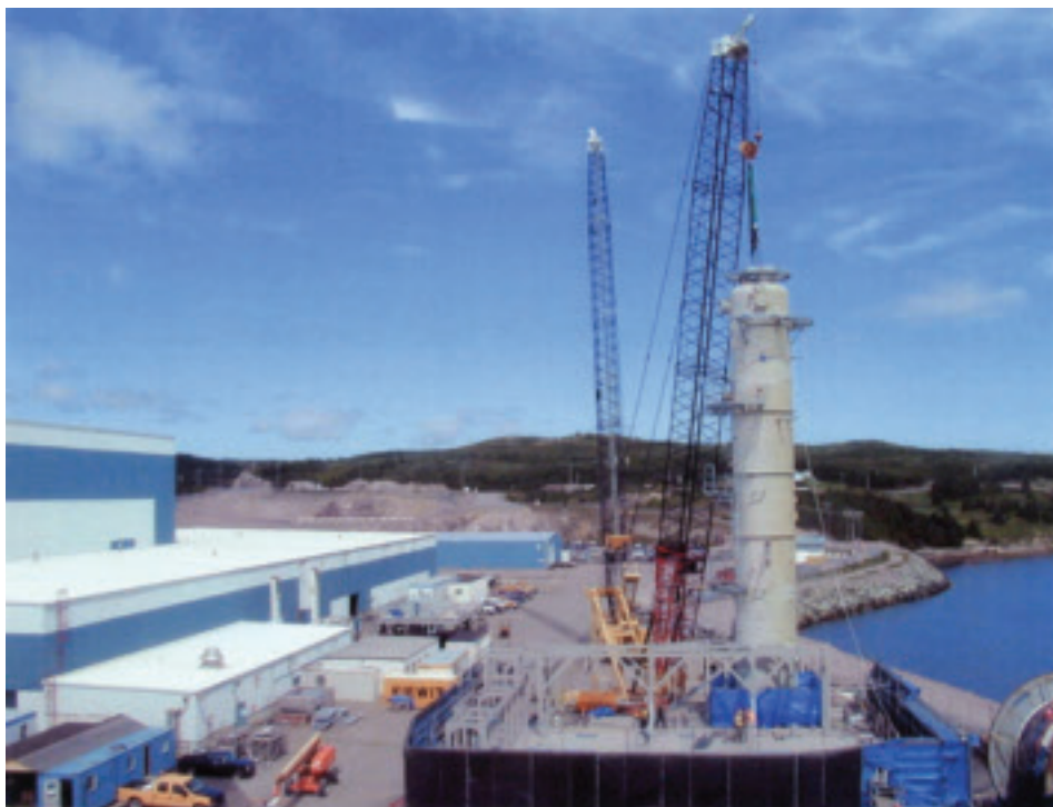
Figure 10: Vacuum deaeration tower. (Courtesy of Eta Process Plant)
